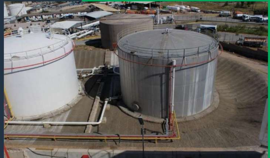
Oil storage protection
